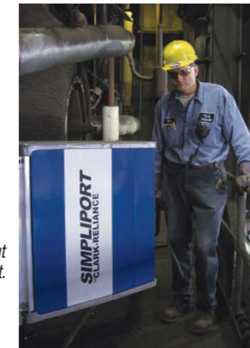
100 year old power plant with Simpliport retrofit.
